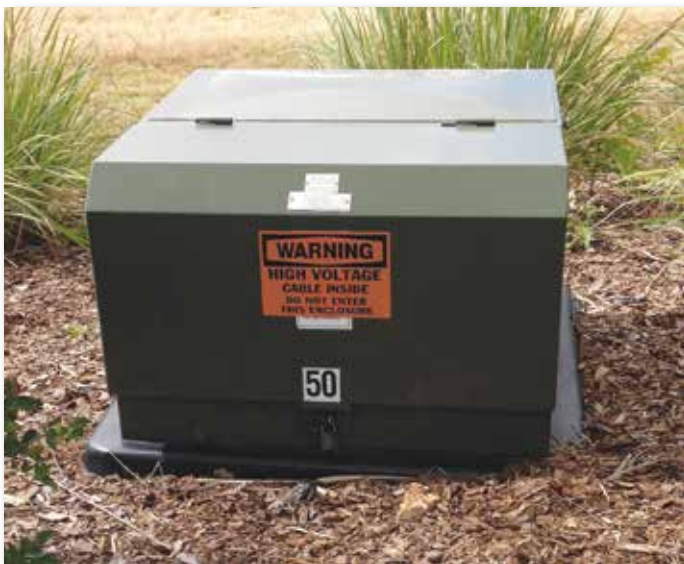
Transformer cabinets are harmless when left alone. Children should not play on or around them. No one except trained OEC personnel should open the cabinets.
