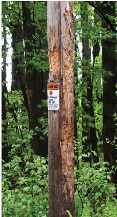
Many utility poles throughout the reservation look like this due to black bears leaving their scent through bites and scratches to mark their territory to other bears. A pole costs approximately $1,500-$2,500 to replace.
