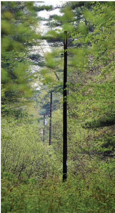
Power lines that run cross country on the MITW reservation. The tribe wants to conserve the land and keep it in its natural state. Overgrown trees are a hazard during storms.
